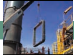
3. GAS TURBINE OUTLET
