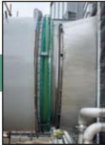
4. DIVERTER INLET 5. DIVERTER OUTLET 1 6. DIVERTER OUTLET 2
